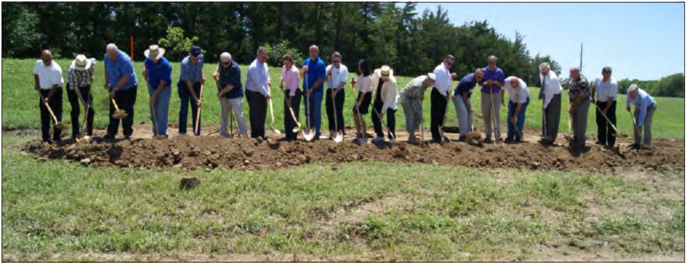
Ground is broken on the Augusta Levee Enhancement project in Augusta, Kansas. The project will raise the height of the levee between two to five feet at various locations and will add another 2,500 feet to the four-mile system.
