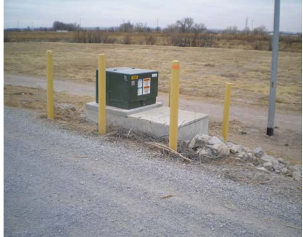
Photograph 2-2. Typical light standard and transformer installation
