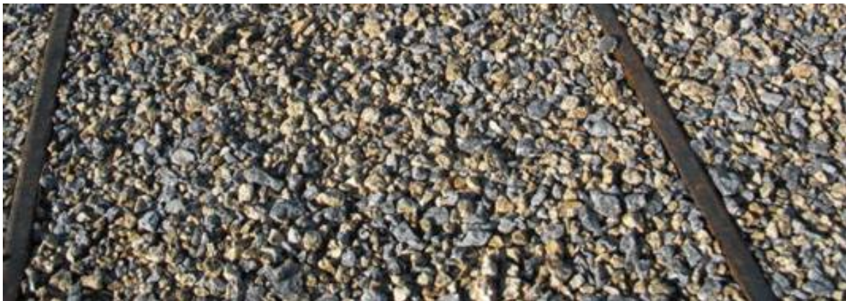
Loose Gravel Between Age Lines
