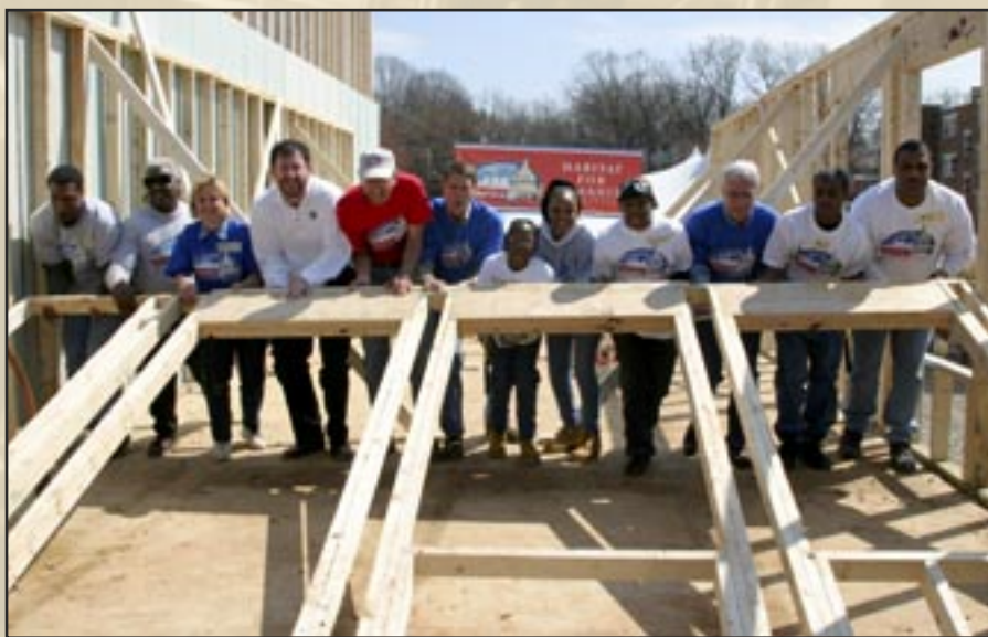
Never a shortage of national service opportunities. A Washington, DC, family welcomed members of Congress who sponsored Congress Building America, a Habitat for Humanity build that resulted in a new home for the family members. Pictured l. to r., raising the frame for a wall are two local volunteers, Sen. Mary Landreiu (D-LA); David Eisner, CEO of the Corporation for National and Community Service; Habitat Founder Millard Fuller; Sen. Bill Frist (R-TN); three members of the Habitat family; Roy A. Bernardi, deputy secretary of Housing and Urban Development; and two other volunteers. Photo courtesy of the Corporation for National and Community Service.
