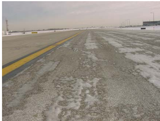
Figure 4. Ice Patches Located on the Test Section, but not on the Adjacent Taxiway, 11/23/04
