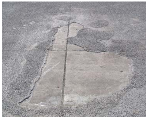
Figure 12. Delaminated Region of the Test Section
