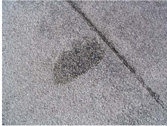
Figure 6. Aggregate Loss at the Test Section Pavement Joint
