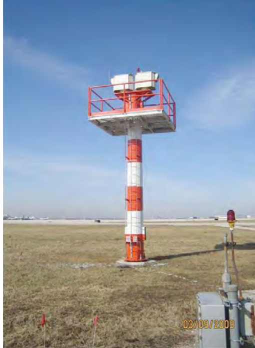
Figure 1. iFerret Sensors Located at ORD Between Runway 27L and Taxiway MM
