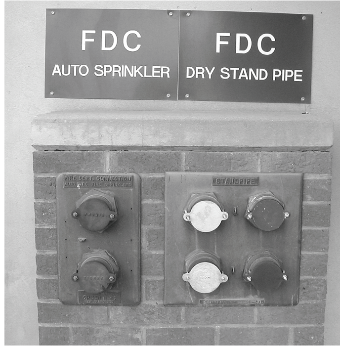
Figure 3-6 Preincident Planning Fire Department Connections Eliminate Confusion
