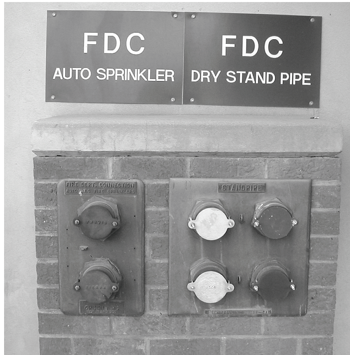
Figure 3-6 Preincident Planning Fire Department Connections Eliminate Confusion
