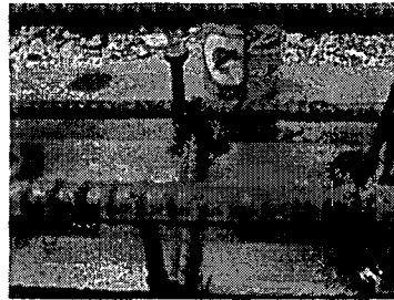
Figure 2: June 3, 2009 Photograph of Closure Strip
