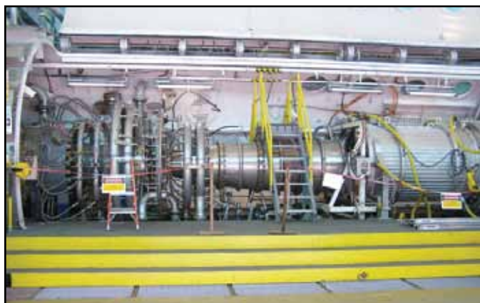
CAH with Freejet Nozzle Installed
