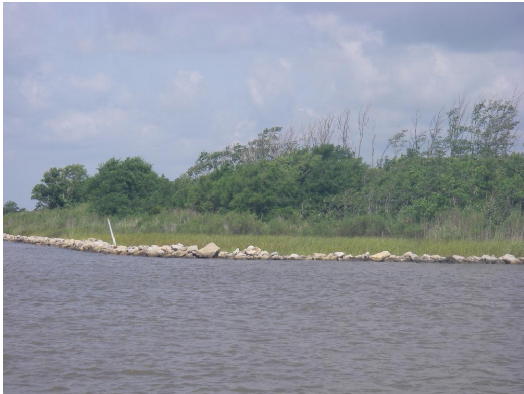
Photo 2. Vegetation behind Rock Dike and damaged settlement plate
