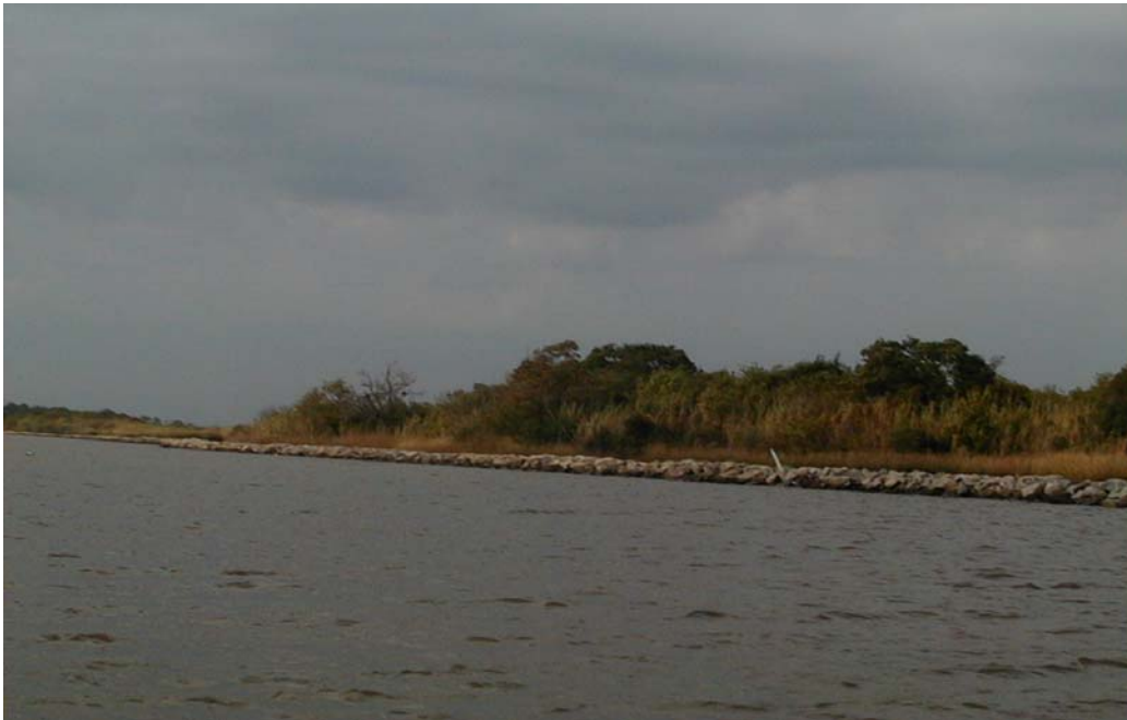
Photo 2—Typical section of dike including damaged settlement plate
