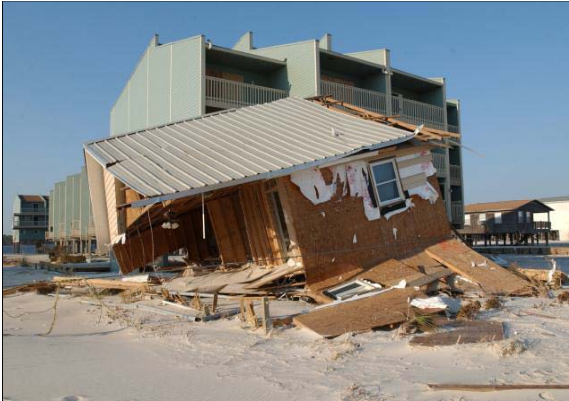
This destruction was caused by Hurricane Ivan as it hit Gulf Shores on the Alabama coast. (Jonas N. Jordan, Savannah District)
