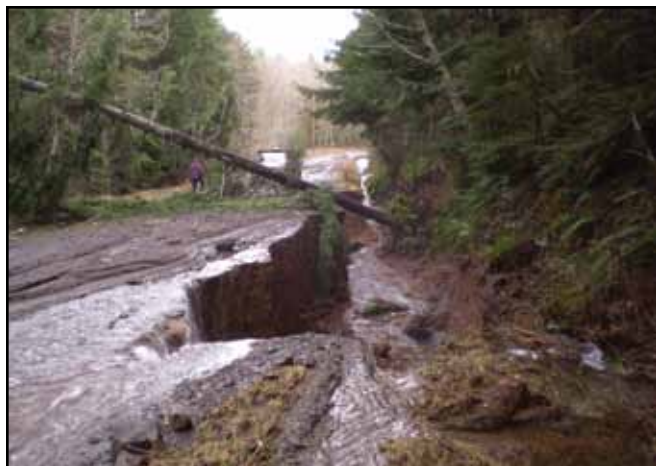
Figure 4.12—Ditch scour along an Olympic National Forest road. Changes in hydrology and physical watershed processes with climate change will likely increase the incidences of culvert capacity being exceeded, fill slope failures, and development of first-order channels that can affect roads and related structures. (Photo courtesy of USDA Forest Service, Olympic National Forest.)
