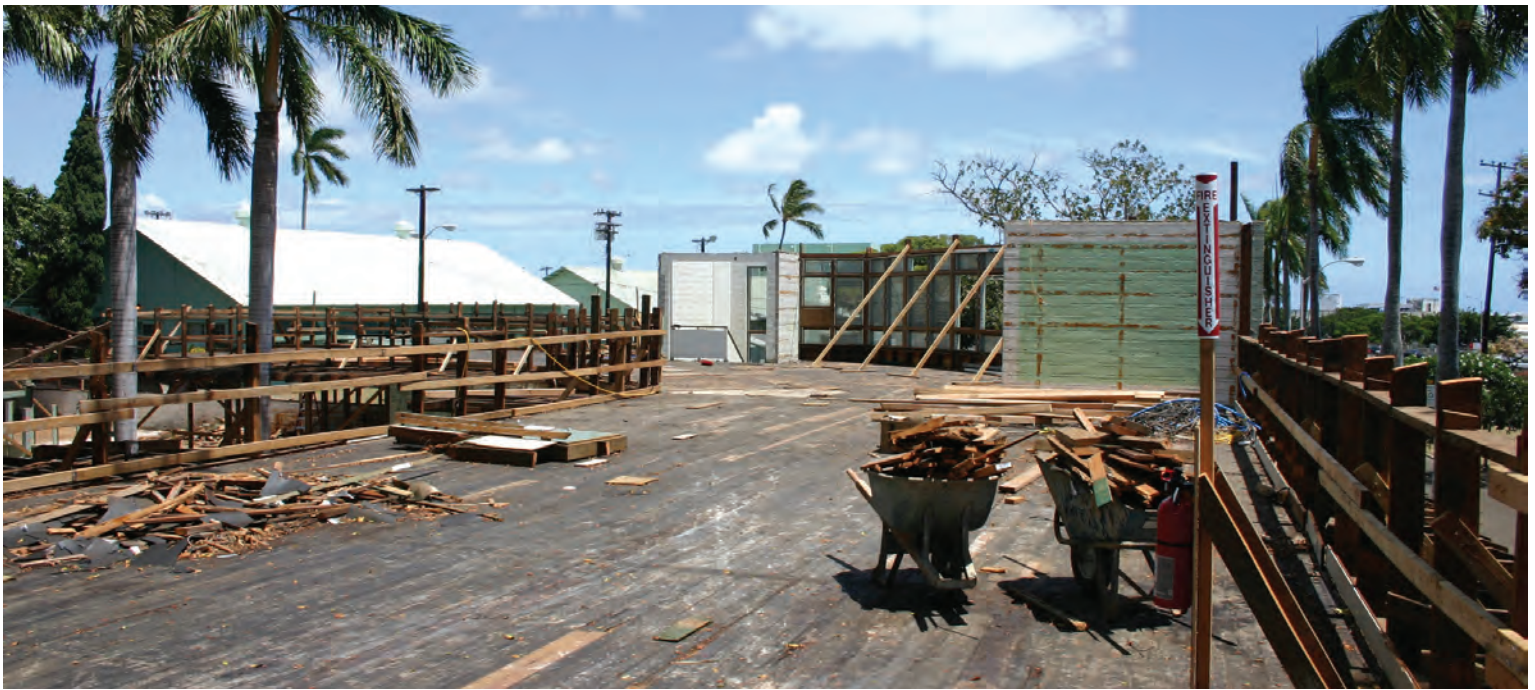
Work crews carefully removed sections of the old Aloha Center - sometimes piece by piece - to ensure the historic integrity of the nearly 70 year-old facility. This view shows the second floor during the debris removal process. Courtesy photo
