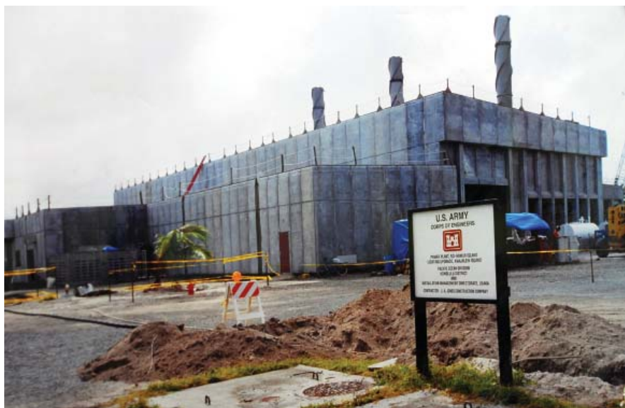
(Top) The Headquarters, U.S. Army Kwajalein Atoll signage shares space with Kwajalein’s “distance-to-home” post. Photo courtesy of USAKA (Middle) San Juan Construction Company, under a Military Construction Army program contract with the Corps, completed construction of the Vehicle Paint and Prep Facility on Kwajalein in 2007. Photo courtesy of Louis Askew (Above) The Corps’ Kwajalein Resident Office oversaw the building of the 13.5 megawatt power plant on the island of Roi Namur. The 34,000 sq. ft. facility houses nine 1,500 kilowatt diesel engine-generator sets with state-of-the-art controls. It was completed in 2001, two months ahead of schedule. Honolulu District file photo
