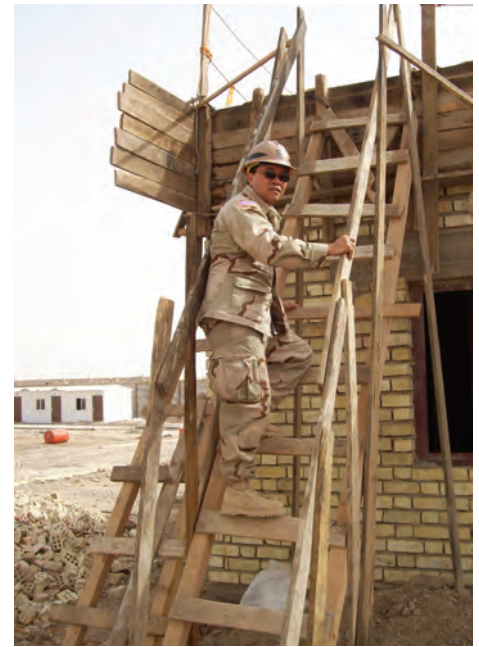
Jon Hosaka prepares to inspect the roof of a dog kennel in the TIFRC under construction near Taji, Iraq. Courtesy Photo
