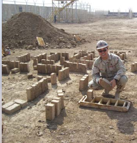
Honolulu District Mechanical Engineer Jon Hosaka shows how to construct hand-made bricks by the use of a simple and ageless process: first pack mortar mix into a wooden form and then dry under the sun. Courtesy photo
