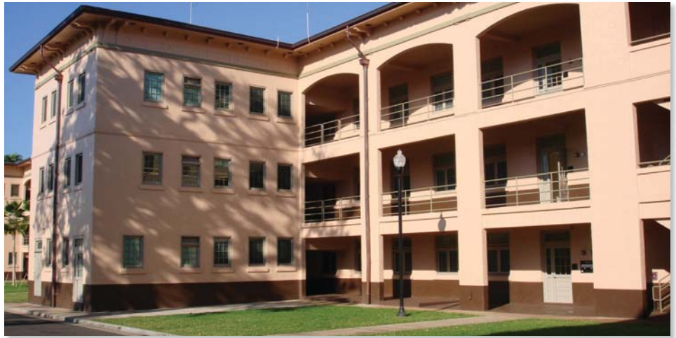
From the lights to the windows to the gutters, Quads C and E have been restored to look like the buildings did in the early 1900s. Photo by Ken Hays, U.S. Army Garrison-Hawaii, Architectural Historian
