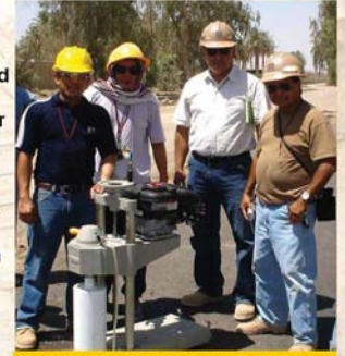
Wayne Birgado (right, in brown hard hat) and crew take a project road core sample.
