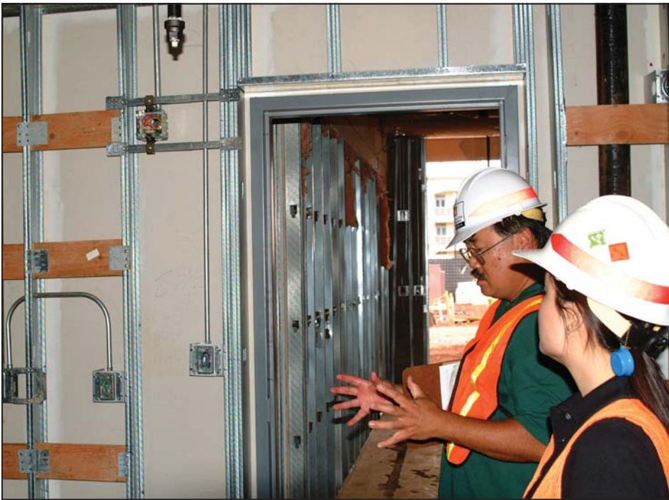
Quad E Project Manager Owen Ogata and Civil Engineer Iris Hew discuss ongoing construction work in Bldg. 551, Quad E. Photo by Dino W. Buchanan
