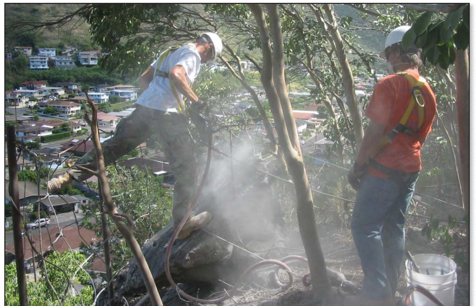
A Prometheus Construction crewman uses a pneumatic splitter to break a boulder on the Tripler slope of Moanalua Valley during the Corps' rockfall mitigation project in late 2005. (Courtesy photo)
