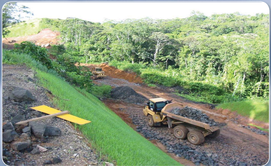
A dump truck prepares to deliver a load of crushed rock for use as a roadbed during construction of the Palau Road in 2004. (Courtesy photo)
