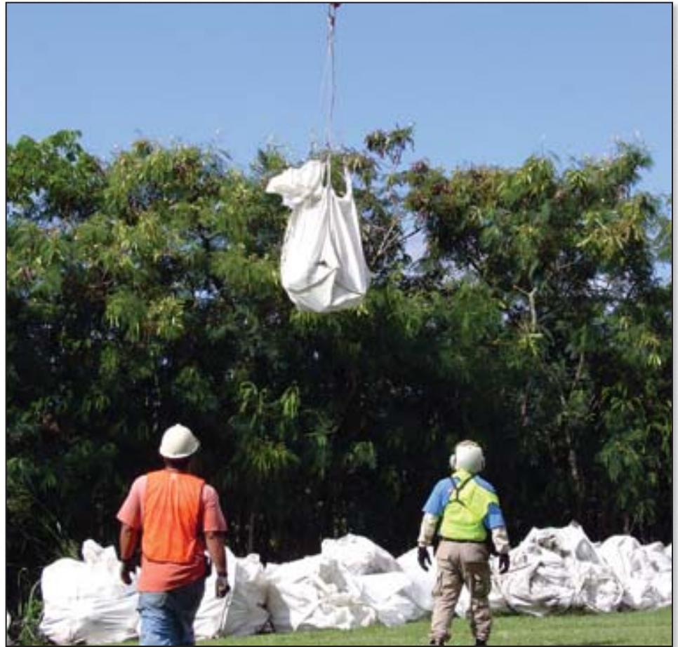
Pacific Aviation and Prometheus Construction workers watch as a bag of boulder fragments is lowered to a field at Tripler Army Medical Center during the Corps 2005 rockfall mitigation project in Moanalua Valley. (Honolulu District file photo)
