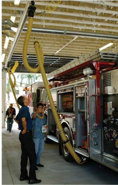
Honolulu District's Andrew Kohashi (left), chief, Army Branch-Hawaii and fire station project manager Tyler Miyamoto (right) examine the fire truck exhaust fume ventilation system at the new Hawaii Federal Fire Station #15 during the grand opening and Hawaiian Blessing held June 15. Photo by Dino W. Buchanan
