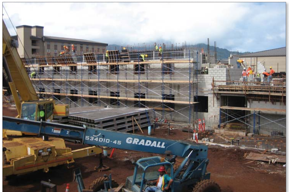
Whole Barracks Renewal (WBR) project Phase 2E at Schofield Barracks is on schedule. The project is part of the more than $900 million WBR Program to upgrade living quarters on Wheeler Army Air Field, Schofield Barracks and Tripler Army Medical Center. When WBR is complete, thousands of Hawaii Soldiers will enjoy modern facilities and improved quality of life. Photo by Tracy Kazunaga
