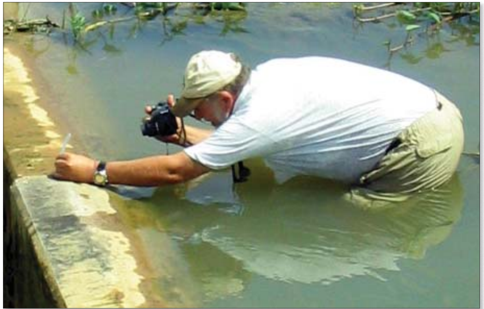
Dan Meyers, Civil Works Technical Branch, documents joint movement and differential head pressures at the weir structure on the federally-constructed and locally-maintained Namu River Flood Control Project, Agat, Guam. Photo by Maj. Robert Kroning
