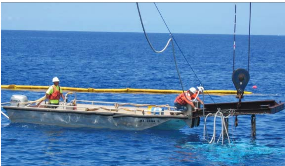
The first Core-Loc is moved into position at Kaunalapau Harbor Aug. 14. When the project is complete, more than 800 of the 35-ton units will be in place. Photo by Paul Mizue
