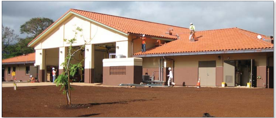
The Fire Station project at Schofield Barracks is scheduled for completion April 2007. Located near Foote Gate, the project will replace the existing historic fire station. The $5 million project will provide a modern and high quality two-company fire station. Photo by Tracy Kazunaga
