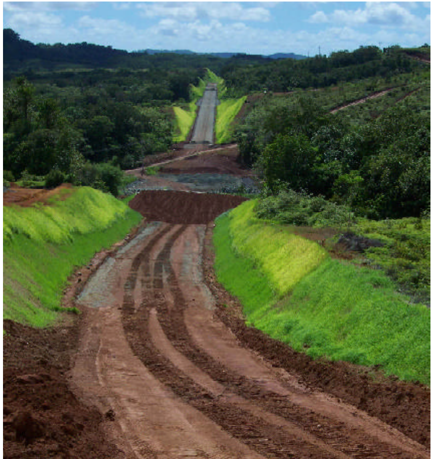
Construction is progressing on the 53-mile long Palau Compact Road. Photo by C. Alex Morrison.
