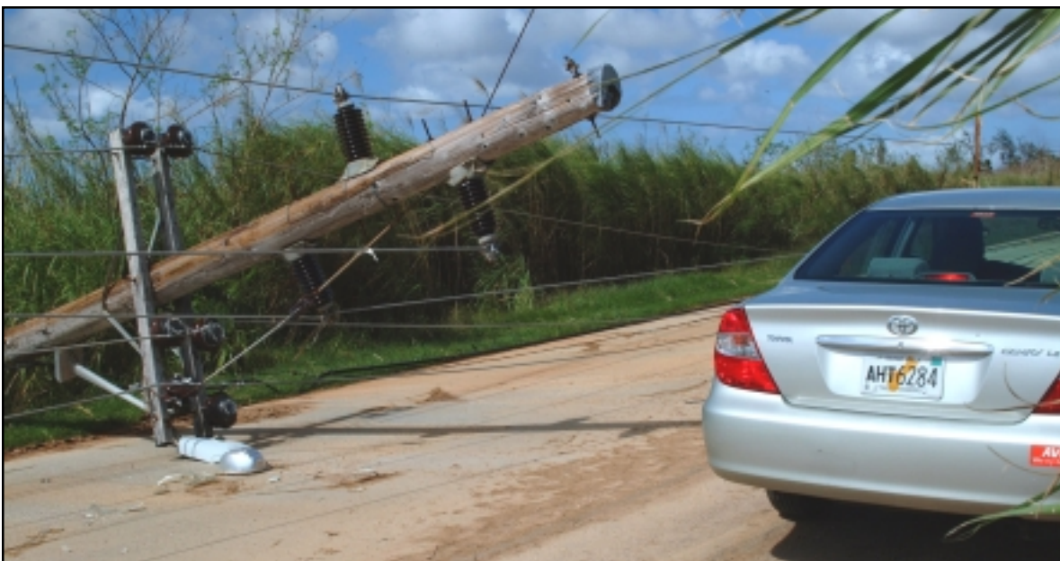
Supertyphoon Pongsona did massive damage all over Guam. Downed power poles are one of the most immediate dangers for drivers, especially at night when they can't be seen from a distance.
