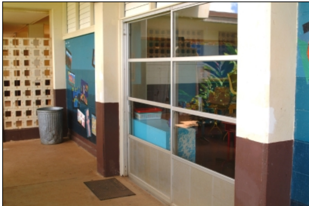
Old doors have been replaced at Mokapu Elementary School, helping to provide better security.
