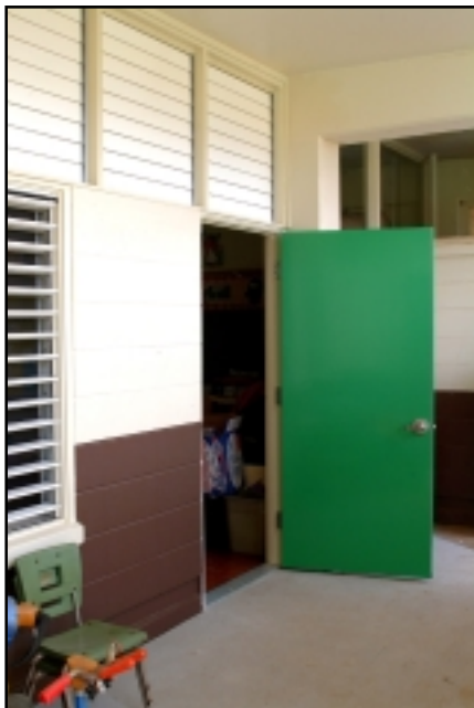
New windows and doors at Mokapu Elementary School make classrooms safer and cooler.
