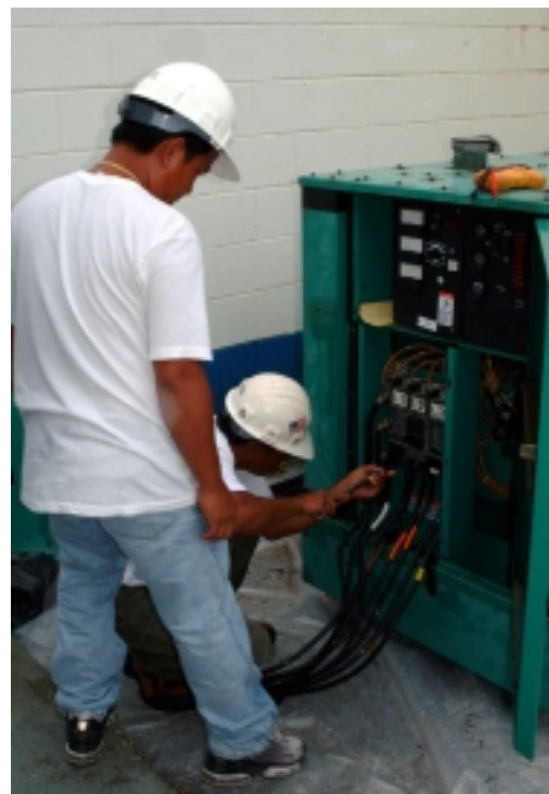
Electricians from Black Construction Company in Guam prepare to disconnect a generator at a school following restoration of the power grid in that area.
