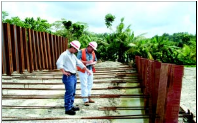
1st Lt. Tom Piazz, pointing, and Mark Wittrock, Palau Resident Office project engineer, check work in Package B of the Palau Compact Road project. Piazz, a recent West Point graduate, was on a temporary duty assignment with HED this summer.
