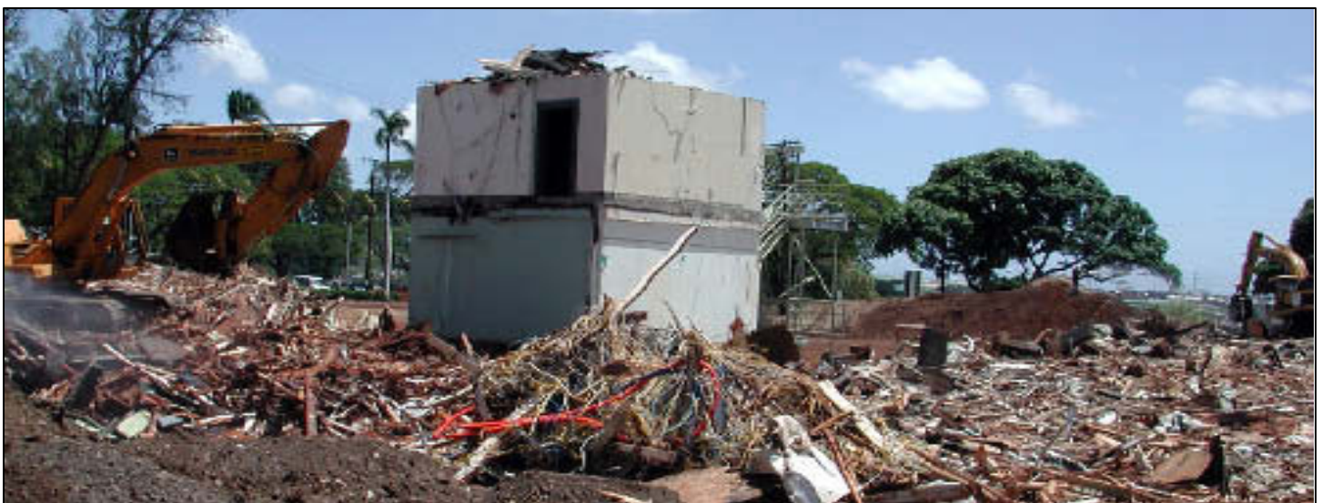
Day Three. War zone or construction site? The two-story reinforced vault is all that remains by the third day.
