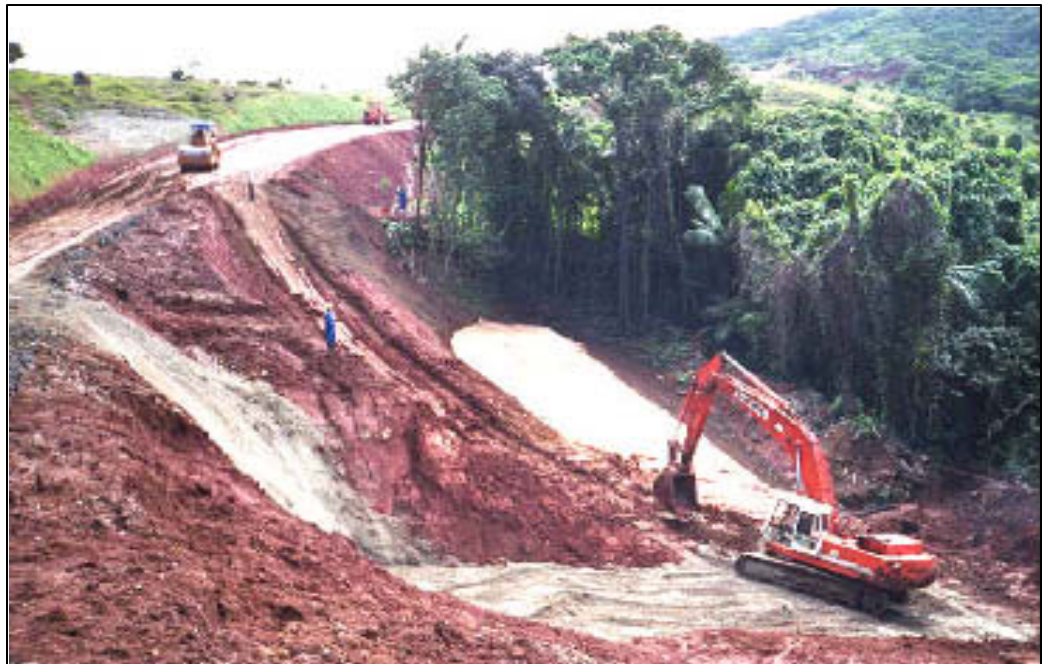
The terrain is one of the factors that makes construction of the Palau Compact Road challenging.
