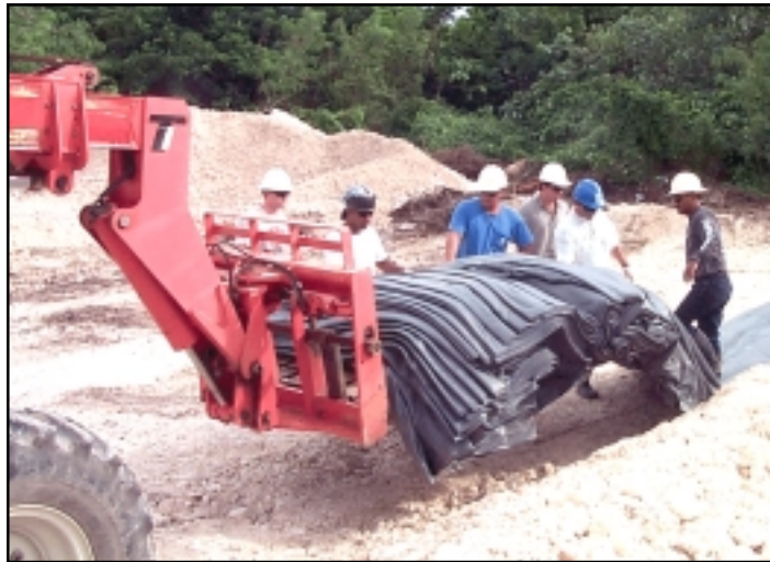
Environmental Chemical Corporation workers place heavy-duty plastic sheeting as they begin constructing a containment cell near the Tanapag Village, Commonwealth of the Northern Marianas PCB-remediation project site. Excavated PCB-contaminated soil will be stored in the cells until the cleanup portion of the project begins. Each containment cell holds approximately 1,500 cubic yards of material. The Tanapag project is one of HED's more challenging Formerly Used Defense Sites cleanup projects and ECC, a leading company in the PCB-remediation field, has been contracted with by the Corps to do the work. — Photo by Frank Ono.
