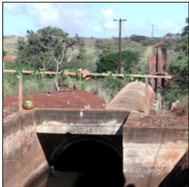
Transmitting water across a gulch, this 85-year-old redwood siphon is soon to be replaced by space-age materials.
