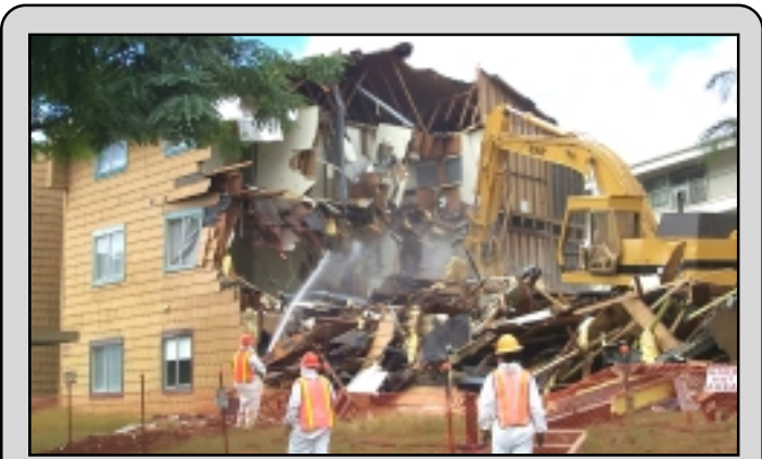
And the walls came tumblin' down... The first of 305 dwelling units scheduled for demolition at Aliamanu Military Reservation came down Nov. 27. The buildings were determined to be too costly to repair due to extensive termite damage and cracks in the foundations. HED awarded the $2.25 million demolition contract to San Construction on Sept. 30, 2000. A second contract for the demolition of 270 additional units at AMR is in the pre-award stage.
