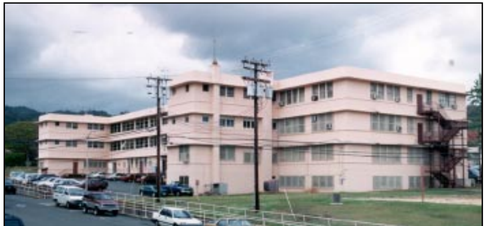
The top floor of building 525 is shaping up to house POD offices. Renovation is complete and wiring is currently being installed for Information Management facilities on a portion of the floor directly below it. From this view the basement of the three story building is visible, making it appear to have four stories. PA photo
