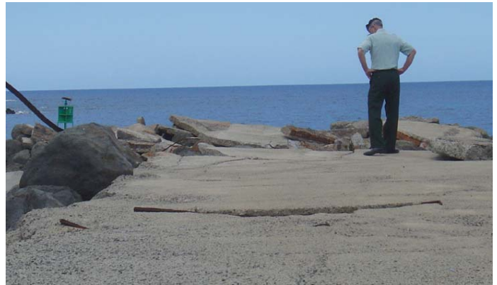
Former POD Commander, Brig. Gen. Larry Davis inspects the existing Kaumalapau Harbor. Courtesy photo
