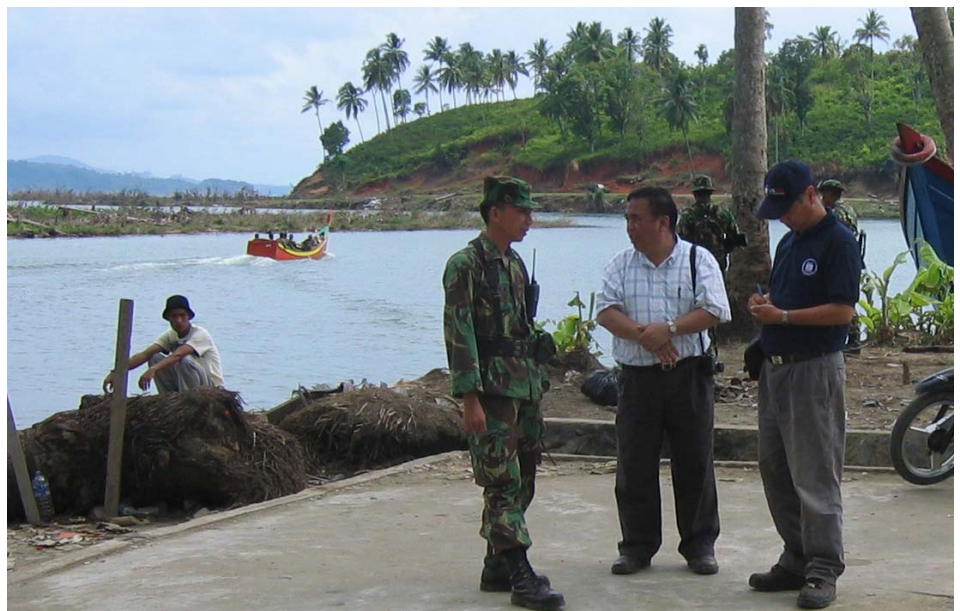
HED Engineer Ron Pang (right) and Edi Setianto of the U.S. Agency for International Development (USAID) discuss damage to the coastal road in Indonesia after the December 2004 tsunami. HED/POD is partnering with USAID to reconstruct the coastal waterway from Banda Aceh to Meulaboh. Courtesy photo
