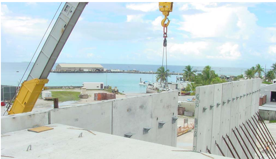
Work is progressing on the $10 million vehicle paint shop on Kwajalein Island. Courtesy photo
