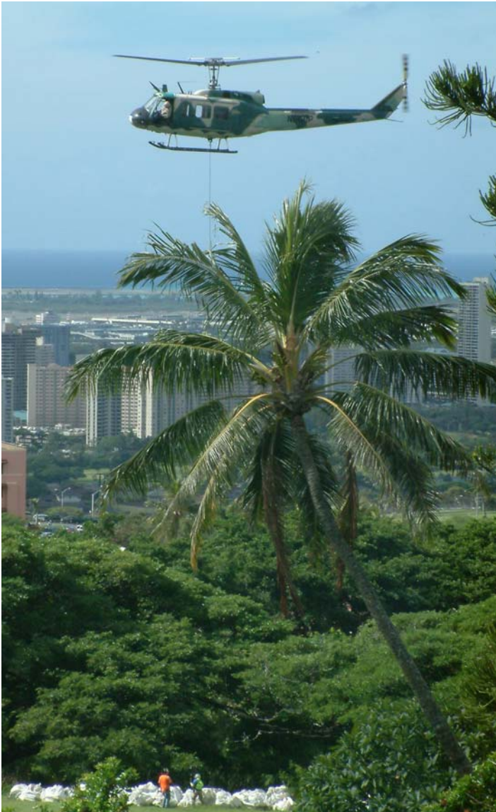
Helicopters removed the remains of approximately 50 boulders from the Moanalua Valley cliffside to a stockpile area on Tripler AMC grounds as part of the Moanalua Rockfall Mitigation Project. HED partnered with the State of Hawaii to prevent potential rockslides to homes in the Moanalua Valley. Photo by Sarah H. Cox
