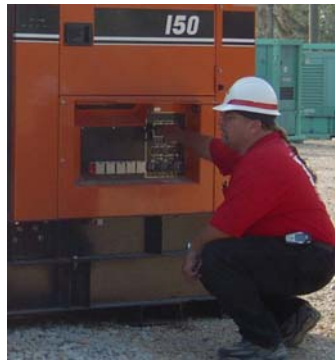
Kennji Santiago (LM) inspects an emergency generator in Mississippi while deployed with the Power PRT. Courtesy photo
