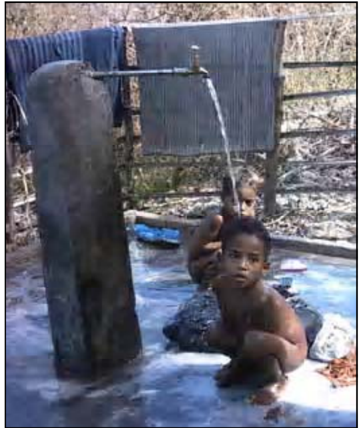
Lotan Village children bathe under one of 12 new community spring water taps constructed by the U.S. Army Corps of Engineers in partnership with local villagers and an East Timor construction company. Lotan Village is located in a mountainous region near the western border of East Timor. Photo by John Emmerson, U.S. Army Corps of Engineers, Pacific Ocean Division.
