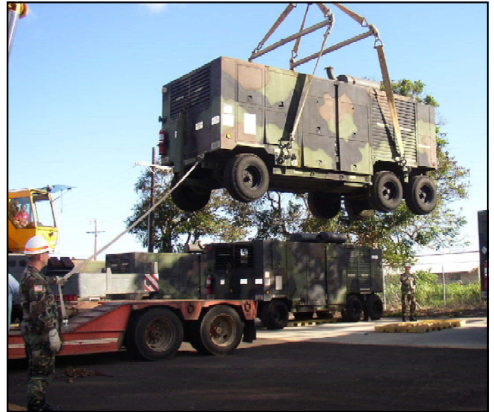
After heavy late October rains knocked out power and flooded 35 of its buildings, the University of Hawaii-Manoa recovered quickly with the support of two electric generators provided by USACE and mission support by the 249 th Engineer Battalion at Schofield Barracks. The military provides cooperative support to the state during disasters as part of a mutual aid agreement and the Joint-Task Force-Homeland Defense and USACE. U.S. Army photo.
