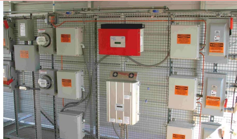
Residential inverters and related disconnects/meters at Sandia's PV Systems Optimization Laboratory
