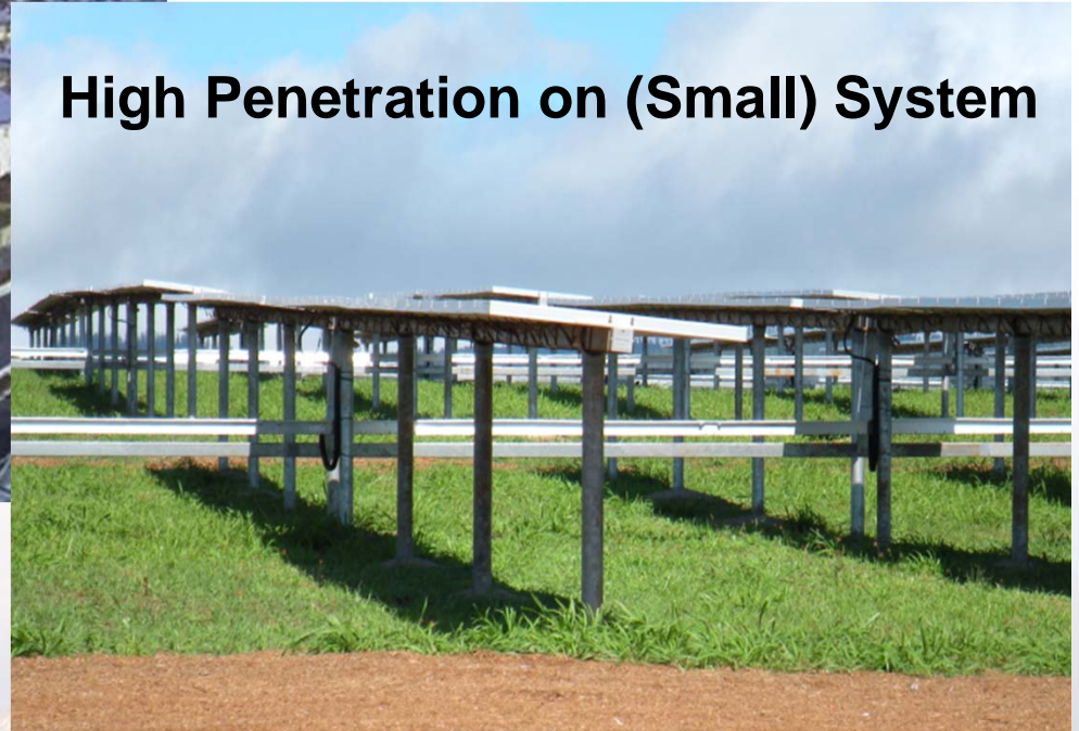
Lanai, Hawaii: 1.2 MW PV system on 4.5 MW island grid supplied by old diesel generators
