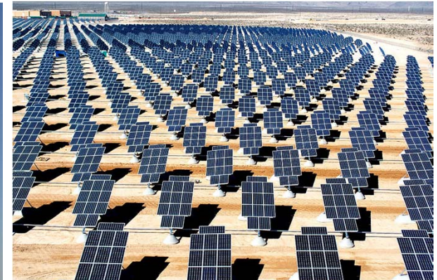
Nellis AFB PV Plant, NV. Photo: Nadine Y. Barclay (GFDL)
