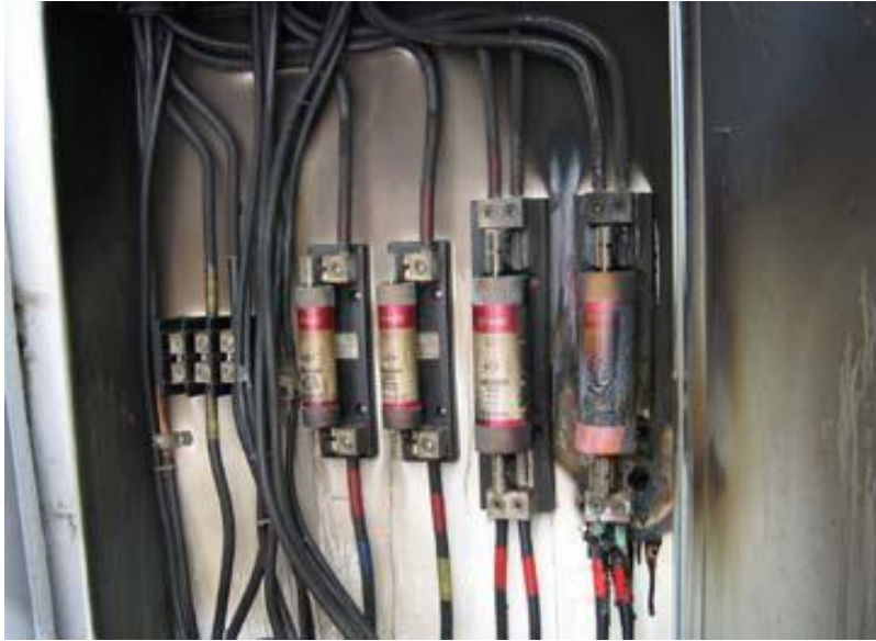
Arcing ground fault
