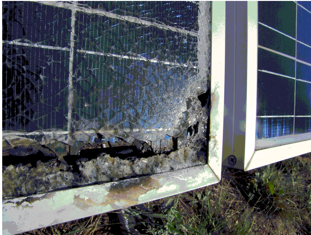
DC arcing to grounded PV metal frame
