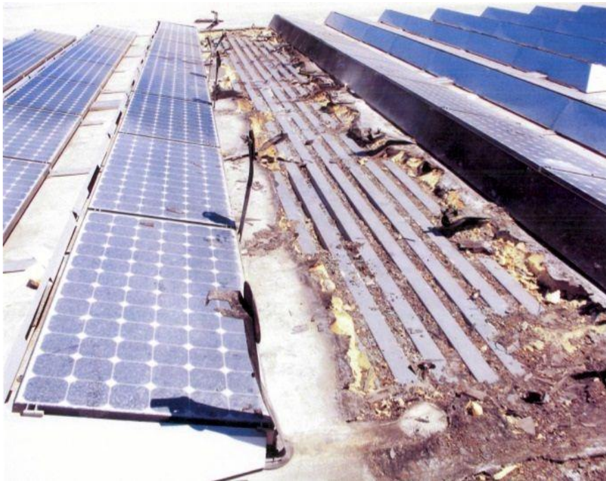
Damage from Arcing Event
