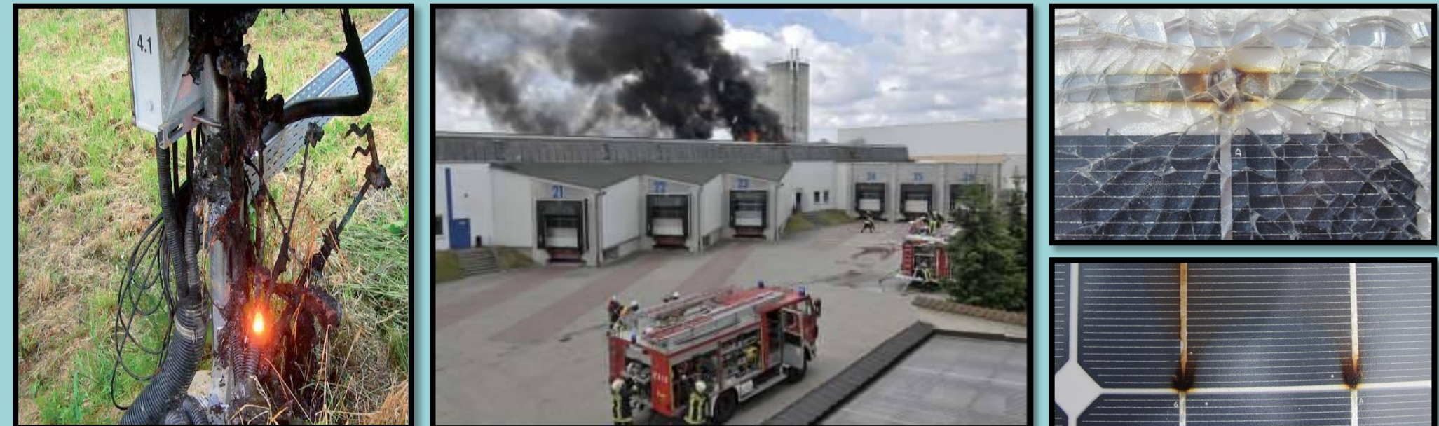
Arcing at the combiner box [1]. PV arc fault-initiated fire on a warehouse in Buerstadt Germany. Discoloration indicating arcing at the busbar and collector ribbon.
