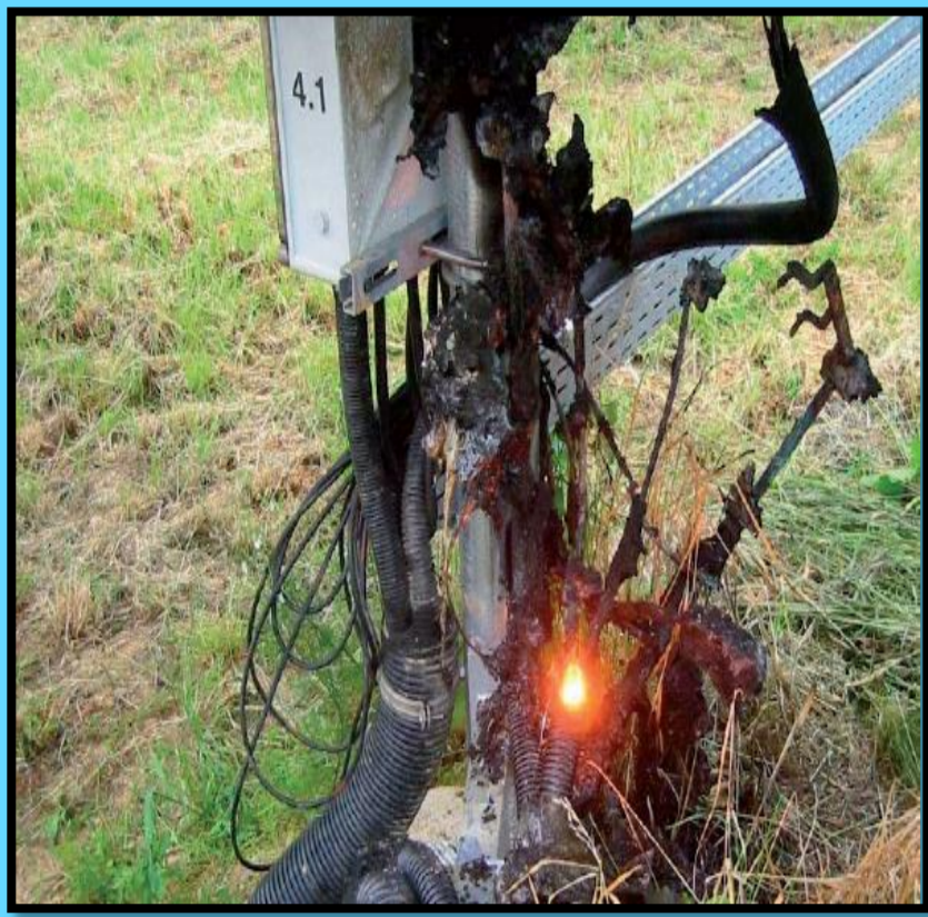
Arcing at the combiner box.
