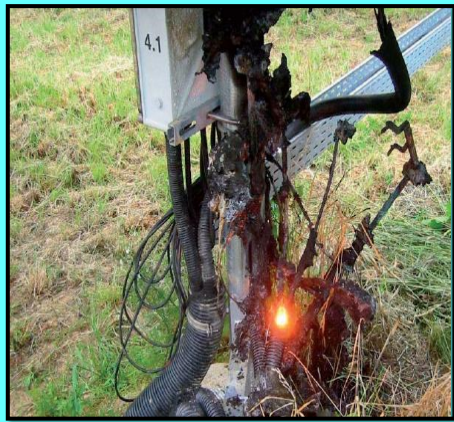
Arcing at the combiner box.
