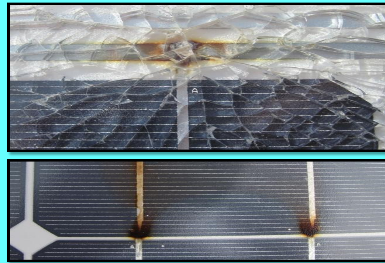
Discoloration indicating arcing at the busbar and collector ribbon.
