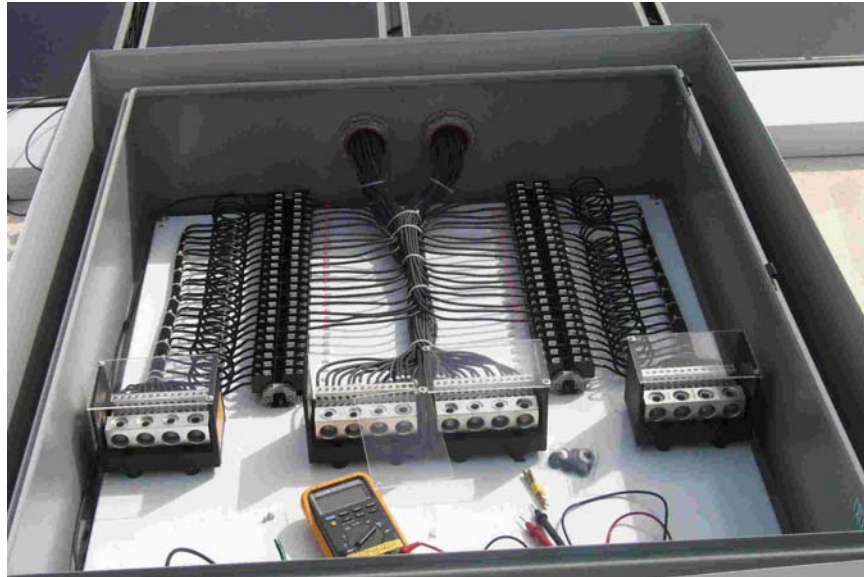
Figure 17. Photo of a wiring ‘combiner box’ housing the terminations for 17 high-voltage module-strings in a large array. In this case, each module string had twelve 150-W p crystalline silicon modules connected in series.
