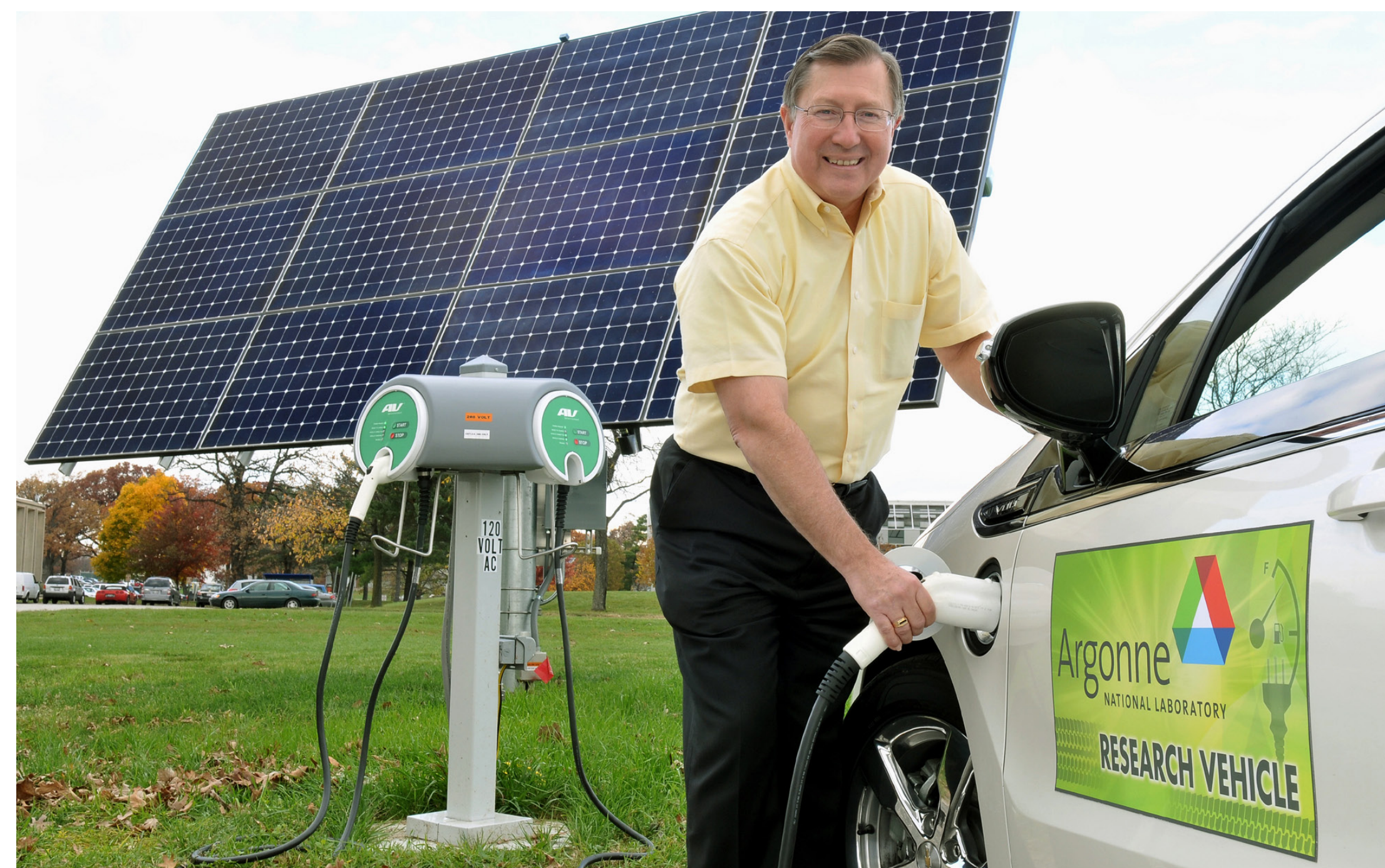
Argonne researcher Glenn Keller charges a test vehicle using the laboratory's solar-powered charging station.
