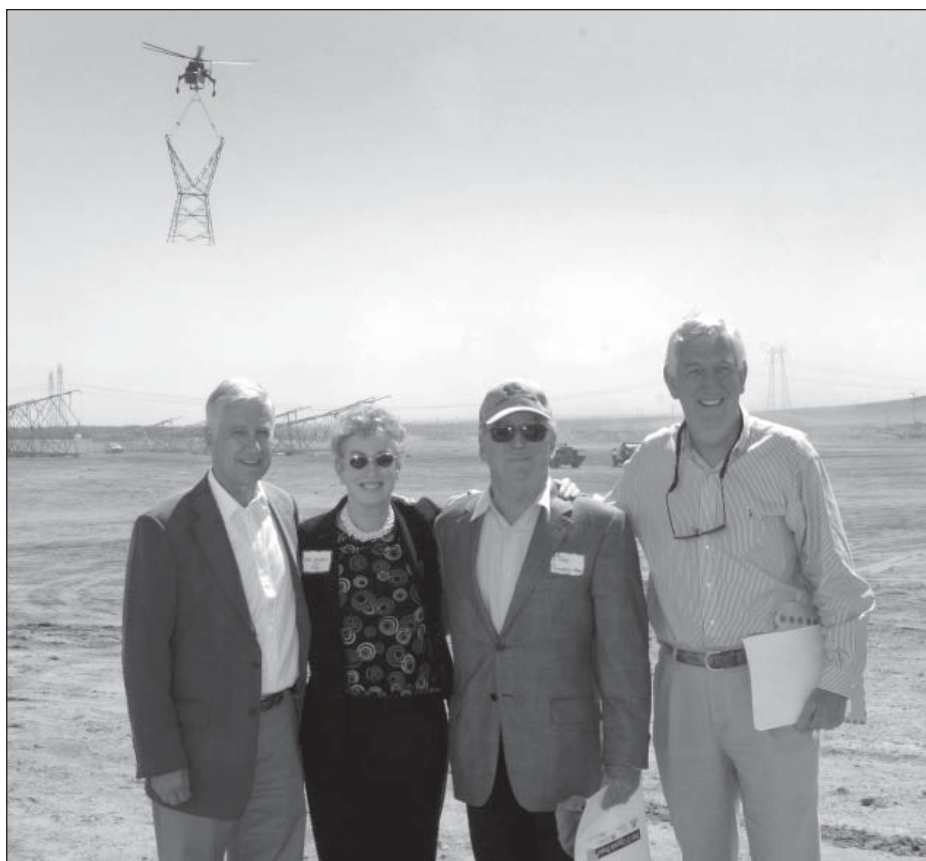
Commissioner Nora Mead Brownell attended a July 2004 event celebrating the expansion of California's Path 15 transmission bottleneck. With Commissioner Brownell, from the left, are Trans-Elect President Robert Mitchell, California Public Utilities Commission President Michael Peevey and Kevin Coughlin, advisor to Mr. Peevey. A helicopter lifts a transmission tower in the background. Photo courtesy Trans-Elect.
