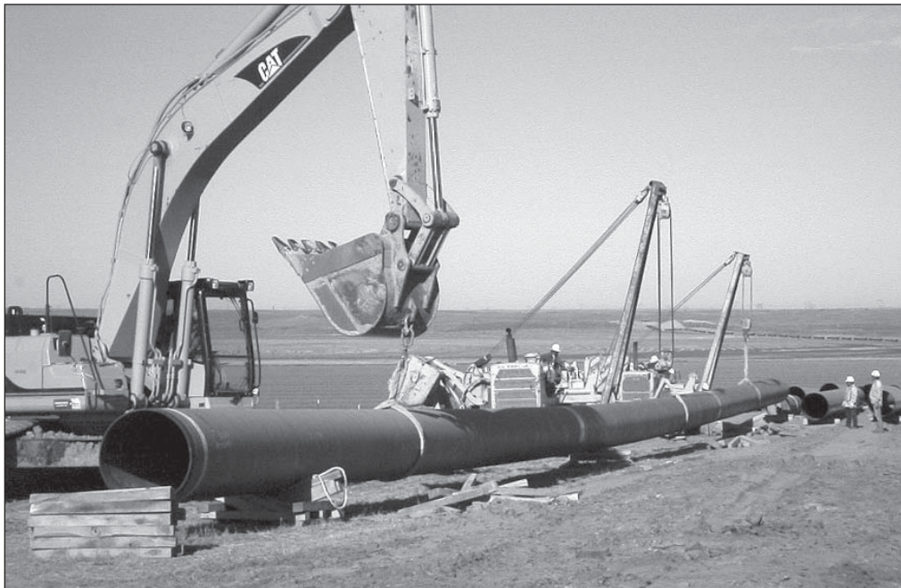
Construction of a natural gas pipeline owned by Cheyenne Plains Gas Pipeline Company, LLC. The 380-mile interstate pipeline begins in northern Colorado near Cheyenne, Wyoming and ends near Greensburg, Kansas.
