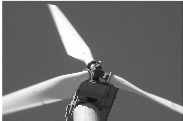
Figure 5. RBU 3 Mounted on LIST Turbine
