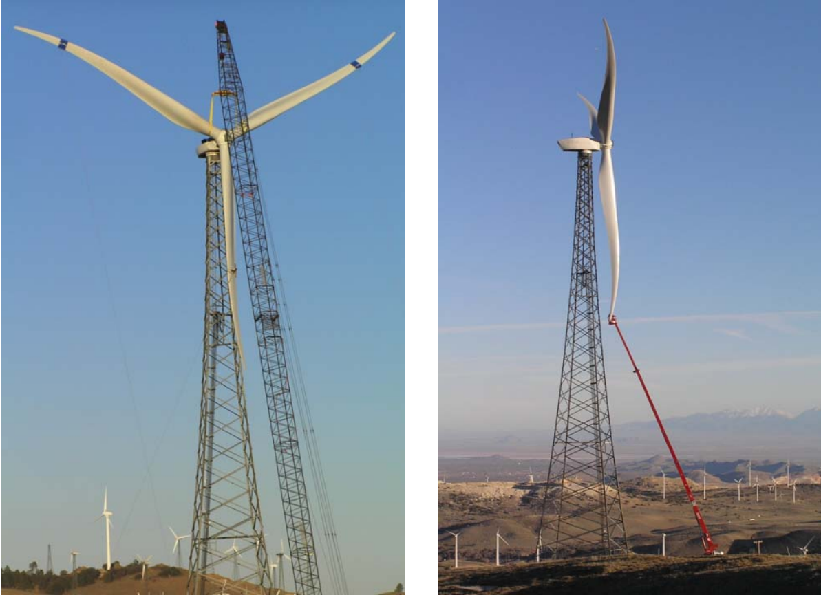
Figure 6.24 STAR rotor during installation and inspection on the RP-09 test turbine in Tehachapi.
