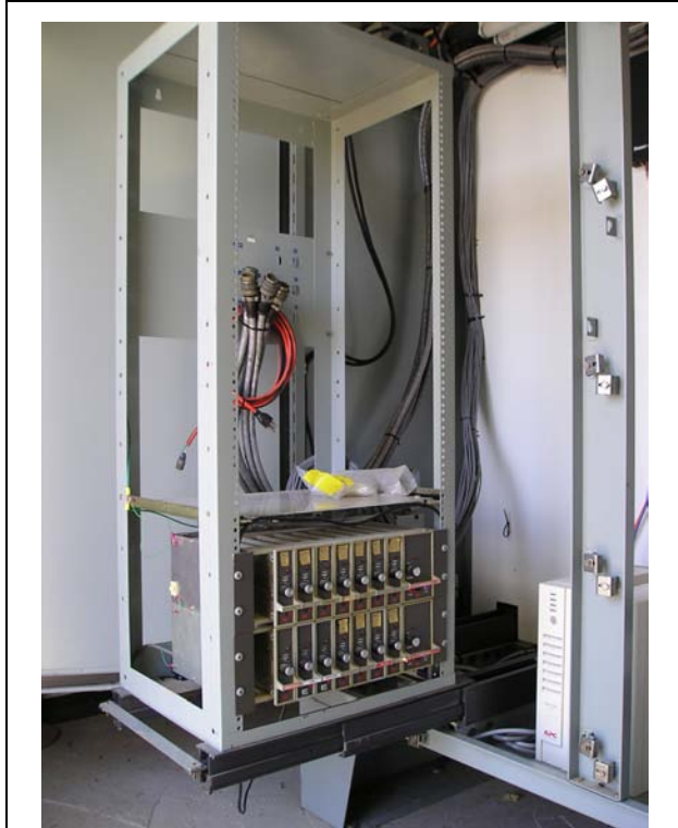
Figure C-5. Front View of the Instrument Rack.
