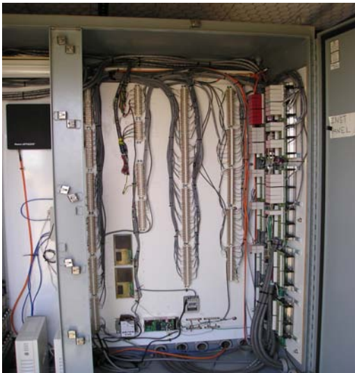
Figure C-1. Power Supplies and Back Panel of the Instrument Enclosure.
