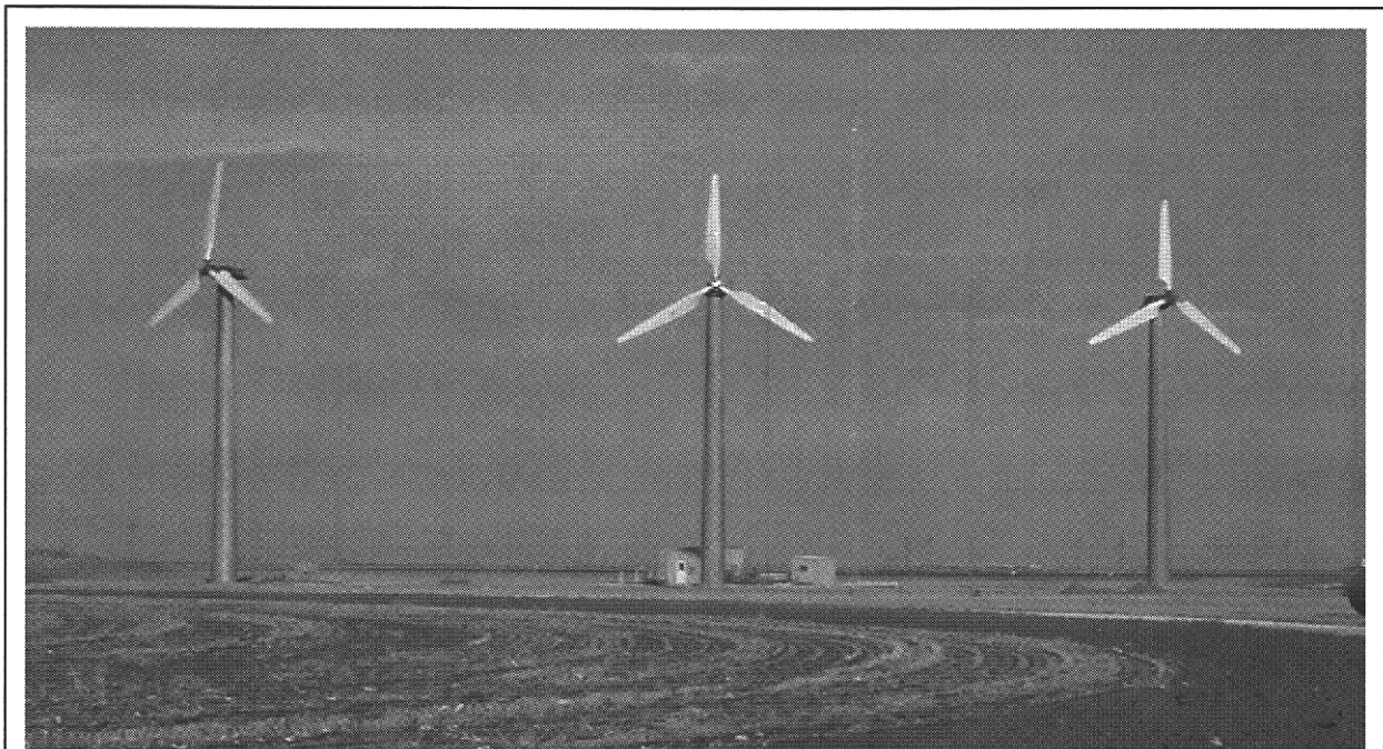
Figure 4. The Test Turbines at the USDA-ARS Site in Bushland, TX.
