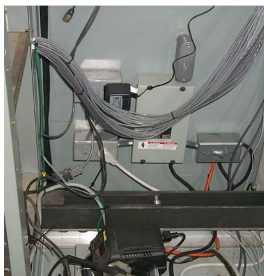
Fig. C-2. AC Power Distribution in the Instrument Enclosure.
