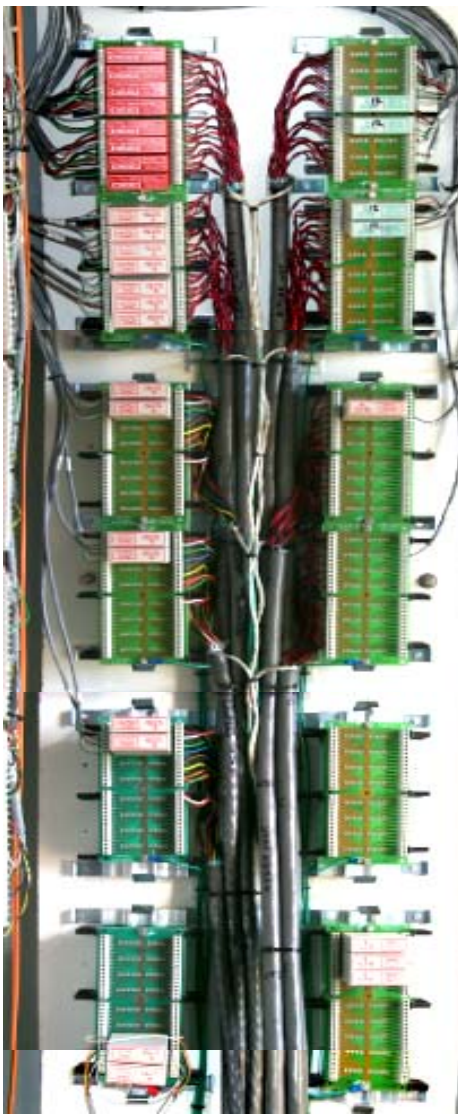
Fig. C-3. Lightning Protection Panels in the Instrument Enclosure.
